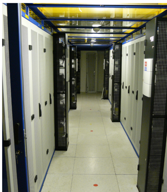
Figure 1: View of server room / optical network installation
