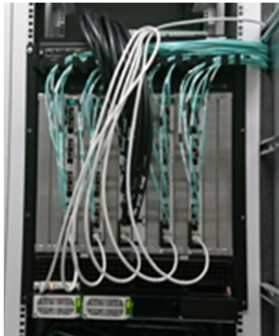
Figure 33: Image of an ATCA crate including train builder and cross-point switch modules to handle data of large 2D detectors. The blue fiber cables connect to the detector and to the further computing systems. The black cables provide high-speed interfaces between the train builder modules. The grey network cables provide configuration, monitoring and control of the train builder system via the control system.
